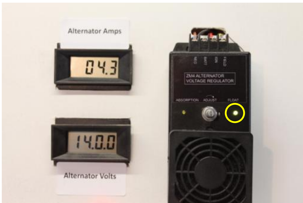
Note: Float phase, Green LED on and battery at 14.00 volts
