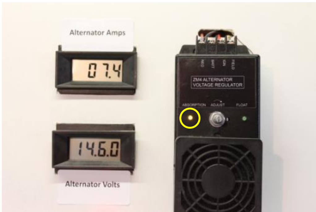
Note: Absorption phase, Yellow LED on and battery at 14.60 volts
